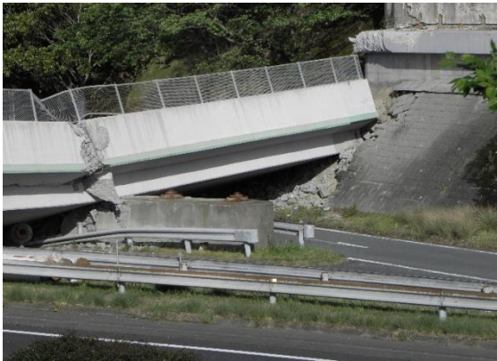
Photo 1 Collapsed bridge near Abutment A1
