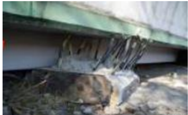
Photo 2 Damage to the displacement confining device
