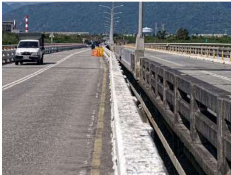
Fig. 1 The lateral deformation of Hualien Bridge[1]
