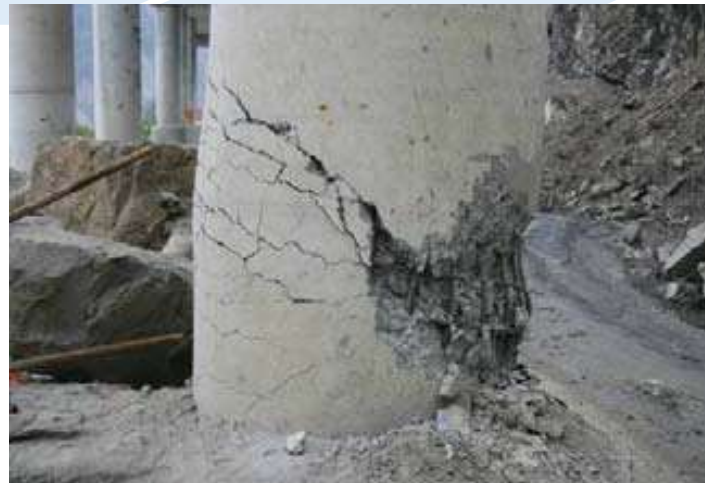
Pier bottom damage
