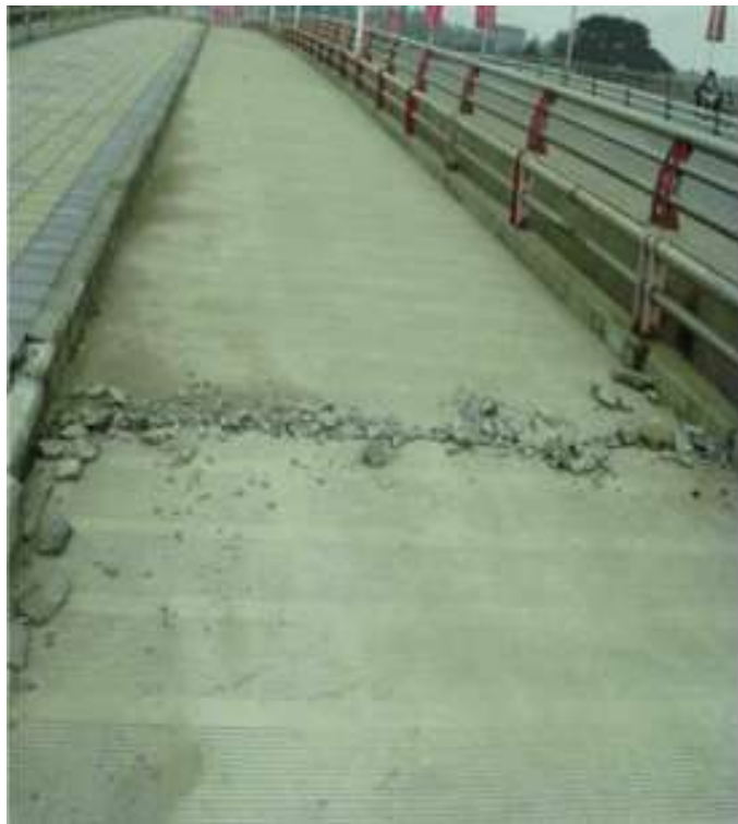
Partial damage of girder
