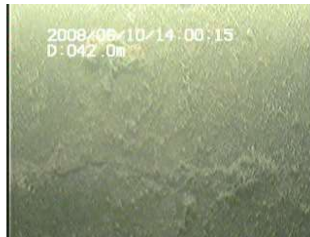
Underwater pier cracks
