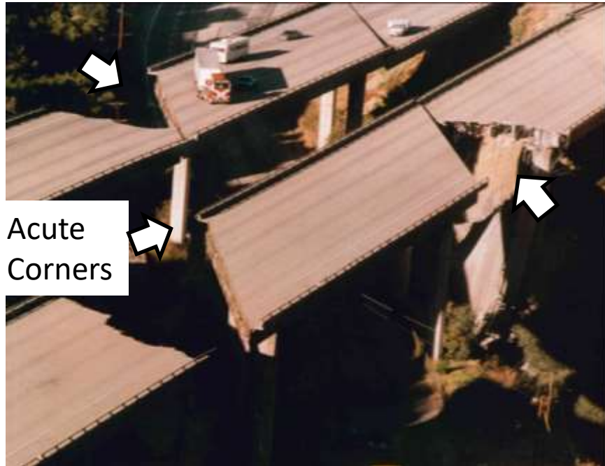
I-5 Overpass at Gavin Canyon (66°) 1994 Northridge Earthquake, CA
