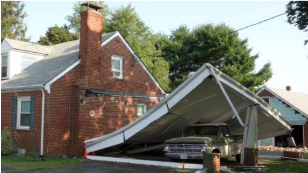
Figure 3. A Carport Collapsed near the Epicenter
