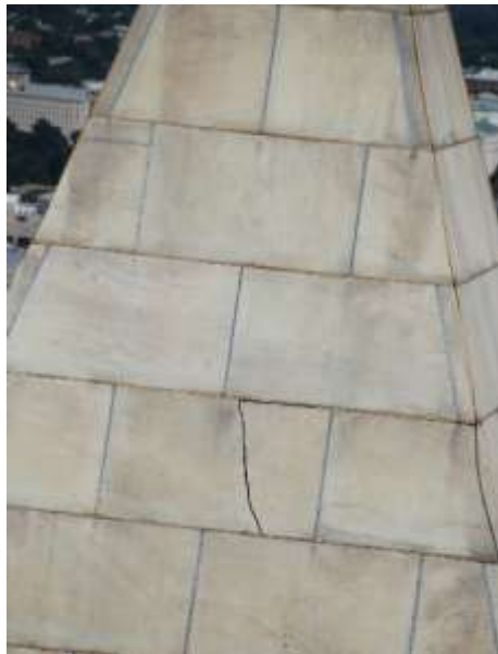
Figure 4. Crack in the Washington Monument
