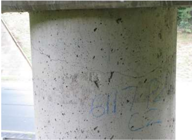
Figure 7. Crack in Column
